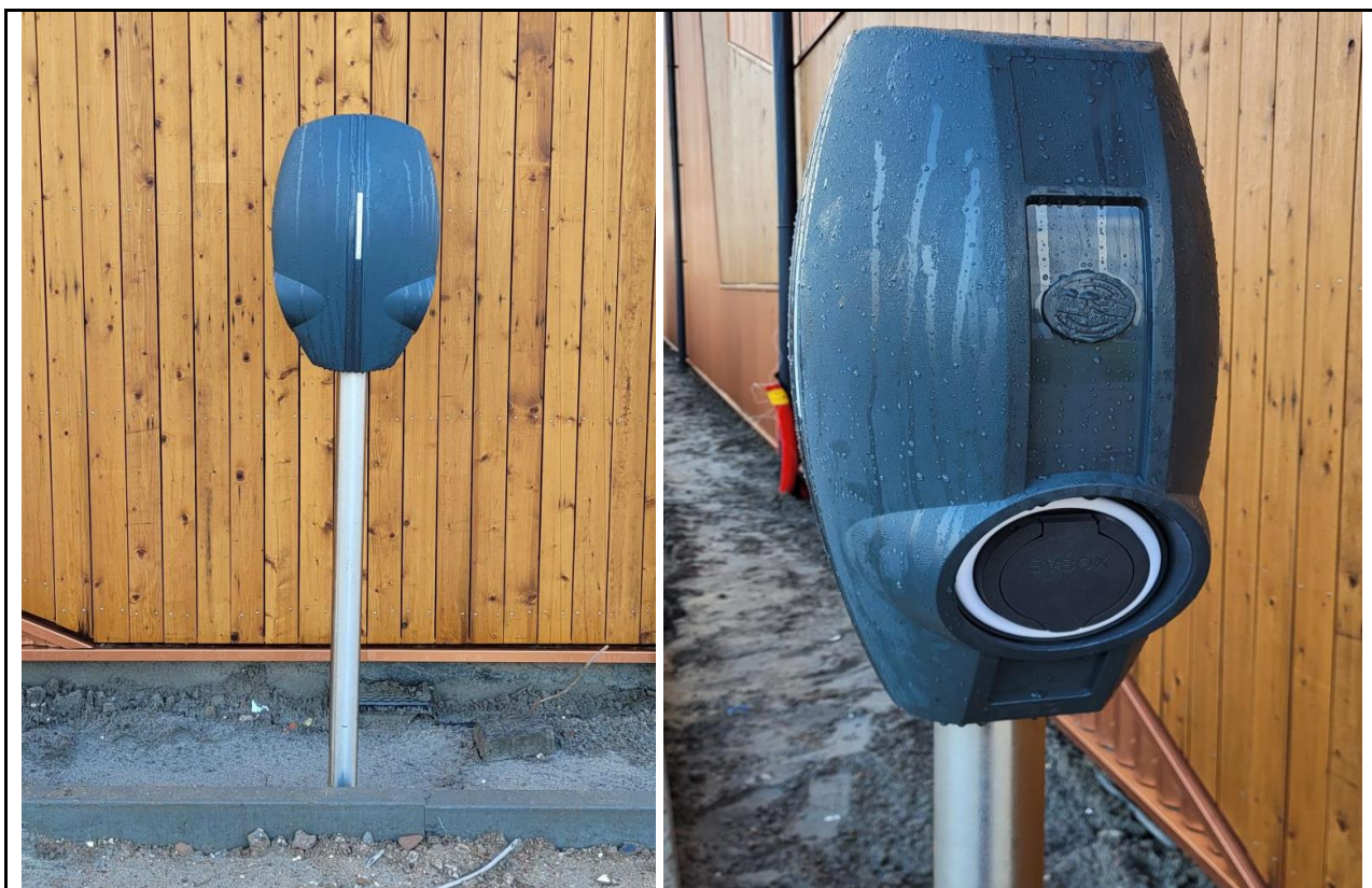
Figure 14: Installed EV boxes at InVesta
