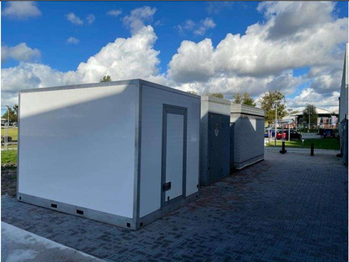
Figure 14: Battery installation at De Meent
