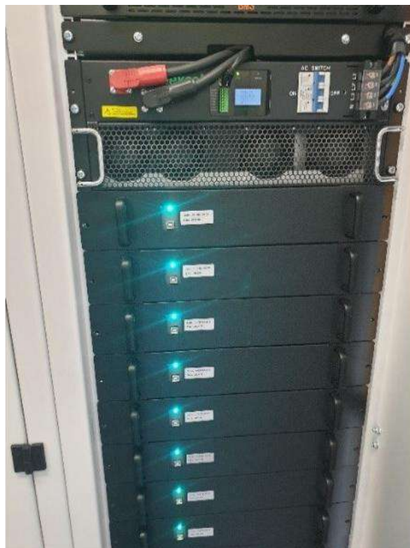
Figure 19: Li-ion Battery at De Meent
