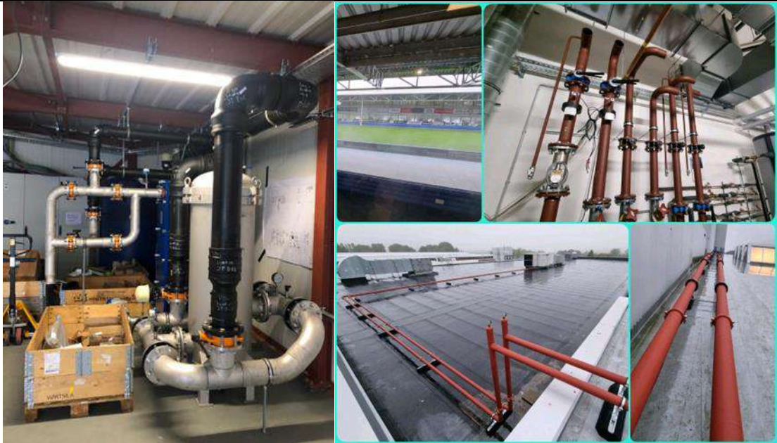
Figure 36: Delivery station and piping
