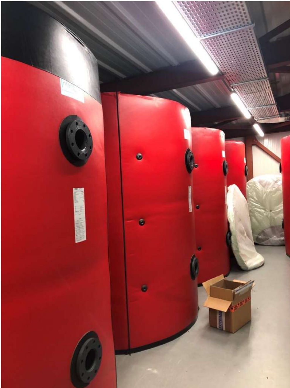
Figure 40: Buffervessels, each 25m 3 for buffering heat
