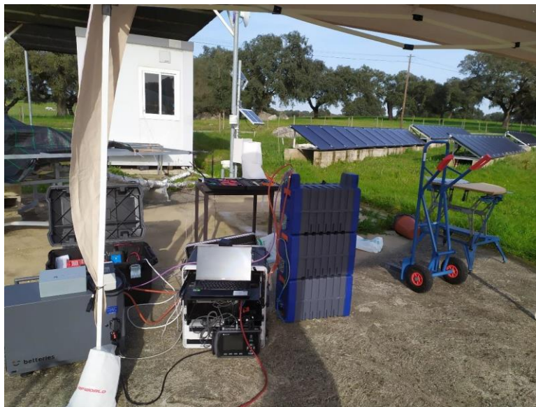
Figure 8 Demonstration of modular 2 nd Life Batteries system in real operation at a fair
